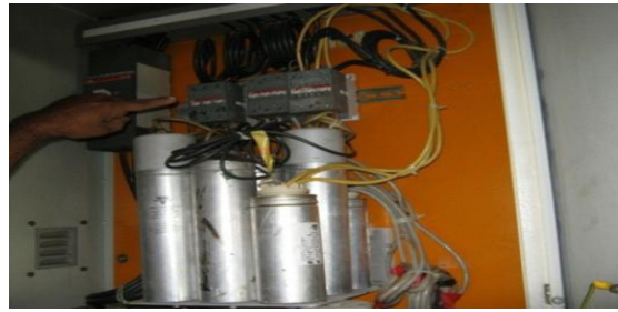
Fig. 2 Power factor correction capacitor for wind generator
