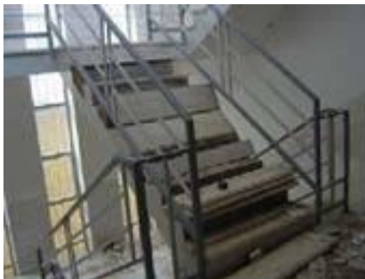
Bam 2003 (Bam Earthquake Report 2003)
