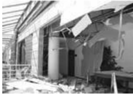
Northridge 1994 (Bam Earthquake Report 2003)
