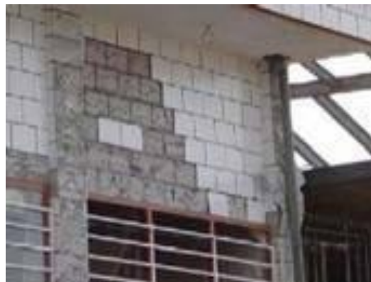
Bam 2003 (Bam Earthquake Report 2003)
