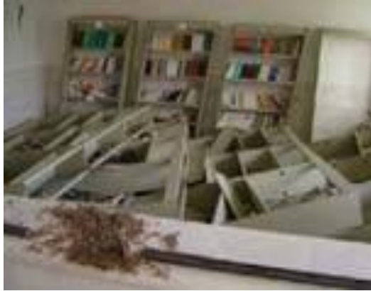
Bam 2003 (Bam Earthquake Report 2003)
