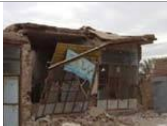
Bam 2003 (Bam Earthquake Report 2003)
