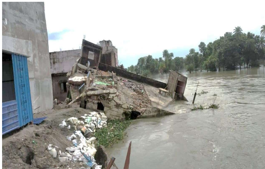
Figure 1.1 The collapse of building constructed near the riverbank
