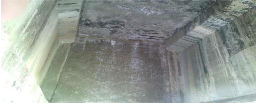
Figure 5. 5 Deterioration in bottom deck slab
