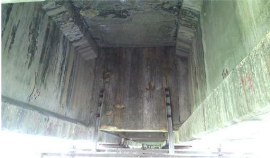
Figure 5. 52 Severe cracks in girder
