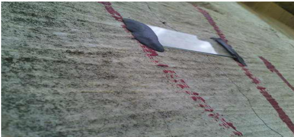
Figure 5. 4 Severe cracks observed in girder
