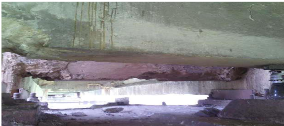
Figure 5. 6 Cracks and delamination at bearings
