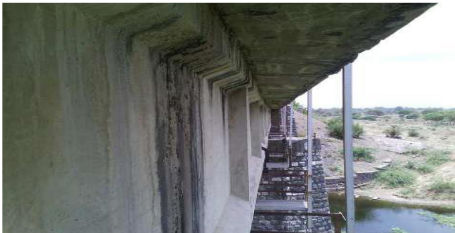
Figure 5. 53 Spalling in diaphragm and girder
