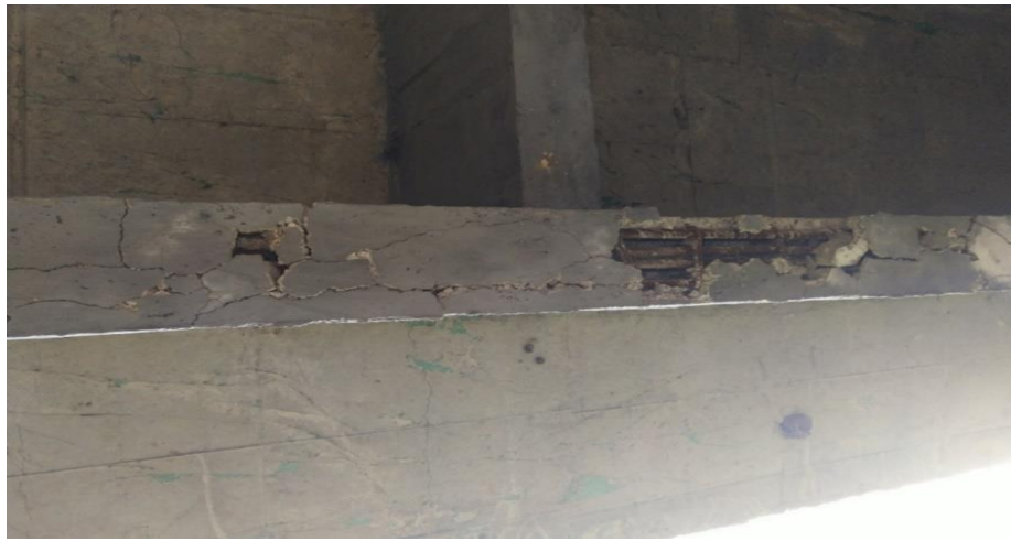
Figure 4. 4 deterioration in bridge girder
