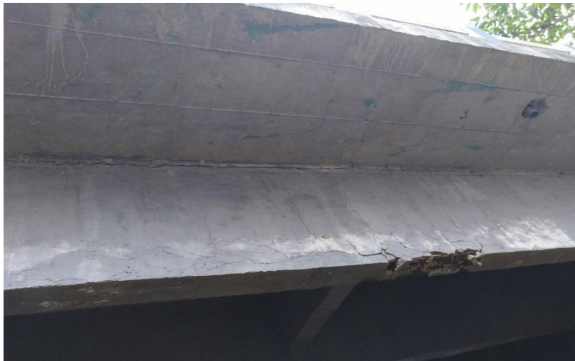
Figure 4. 3 Wide flexural cracks in the full depth of RC girder
