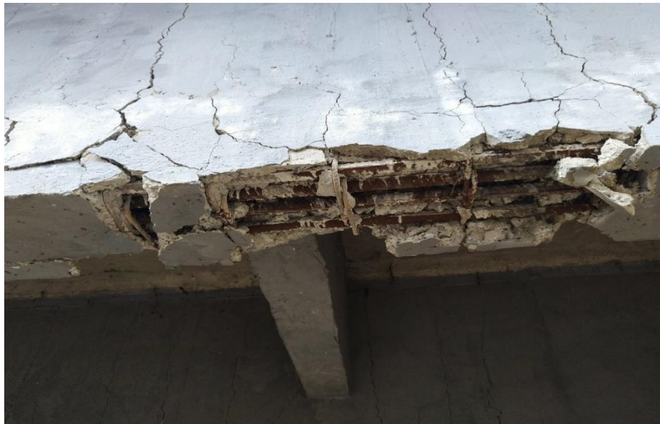
Figure 4. 5 Exposed reinforcement of girder with shear and flexure cracks
