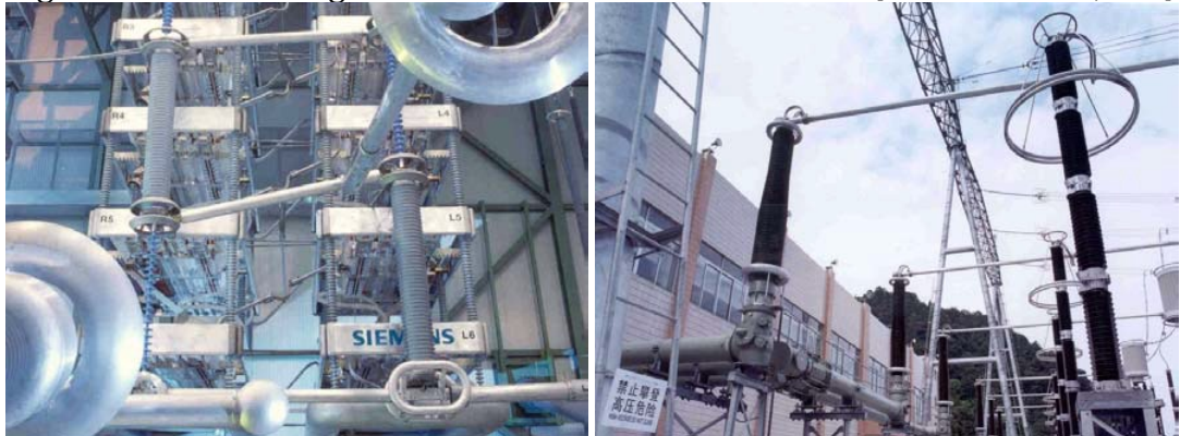
Figure 1.10: Examples of B (left) and A arresters (right) in a HVDC station [CIGRÉ Publication 33/14-05]
