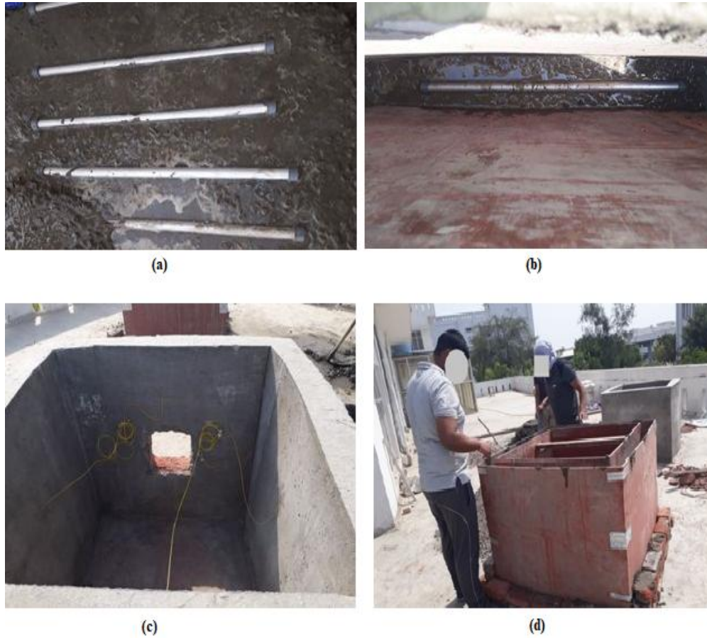
Figure 3.3 Various pictures of the experimental site during the construction (a) Embedding MPCM on the roof (b) Embedding MPCM in the wall (c) Installations of thermocouple inside the cubicles (d) Photograph of the construction site
