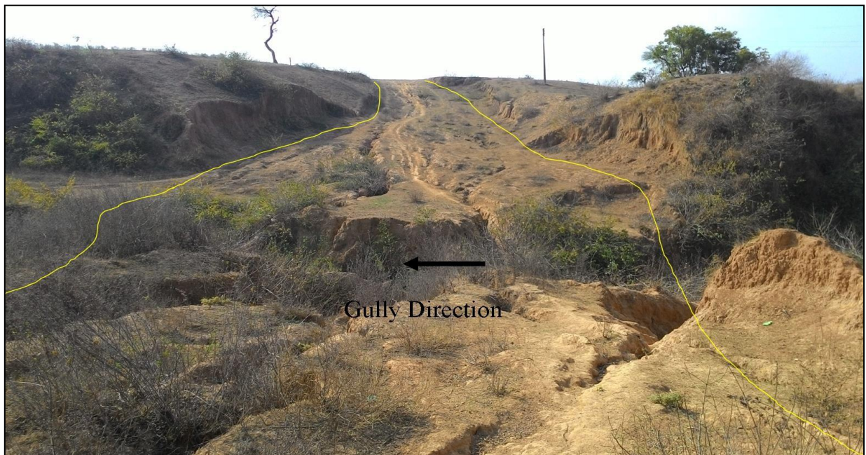
Figure 4. 5 Field photography showing eroded road due to the rejuvenation of a gully
