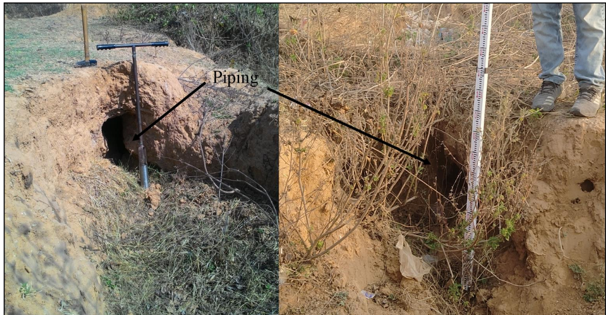
Figure 3. 5 Field photographs showing piping features in the badlands area
