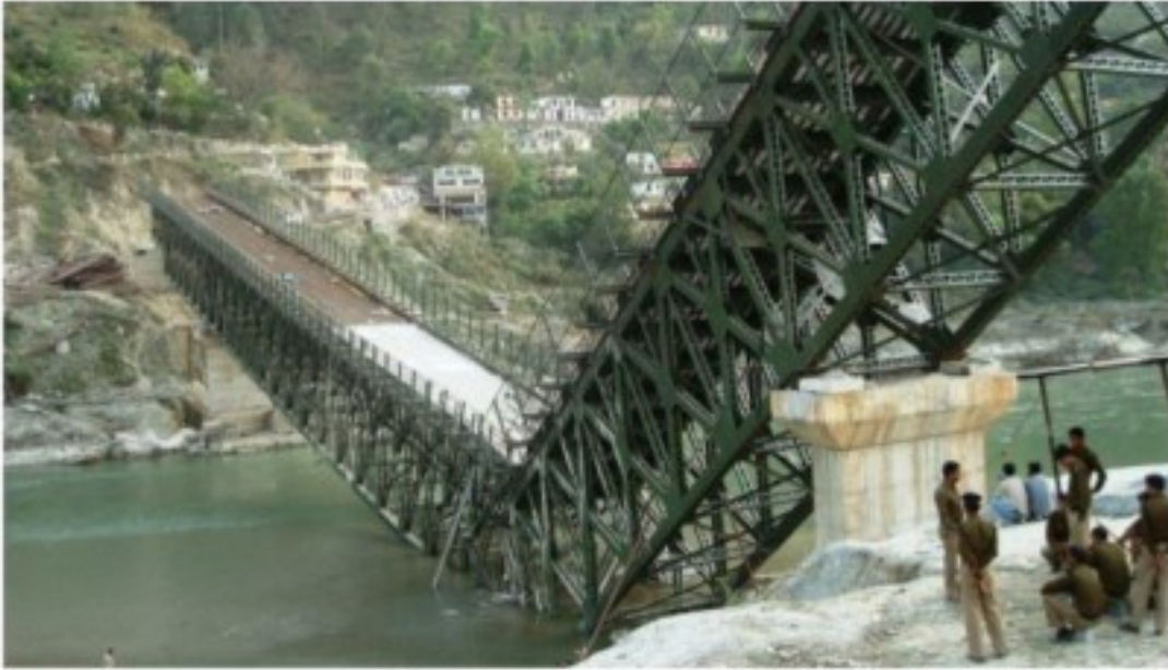
Figure 2.9 Failed Chauras bridge during concreting. [H.S.Birajdar et al., 2014]
