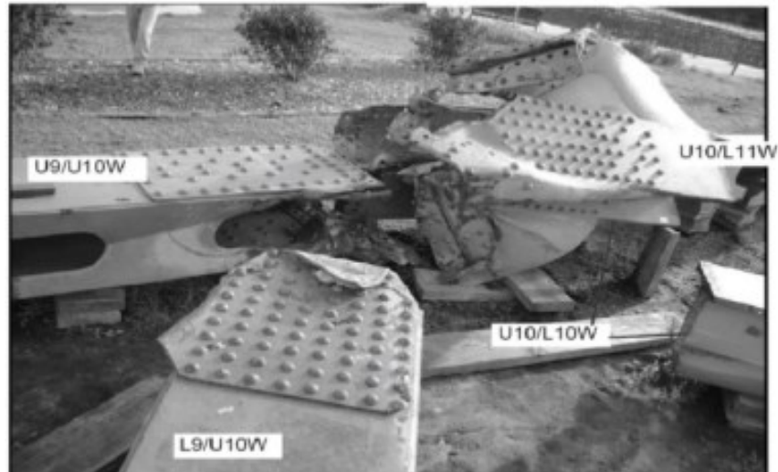
Figure 2.8 Failed gusset plate at U10 joint [M. Liao et al., 2011]
