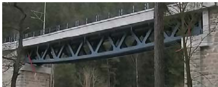
Figure 2.2 Simply supported composite truss bridge of span 36m (J. Machacek, et. al. , 2011)
