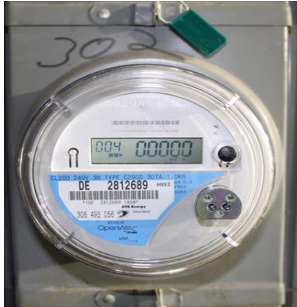
Fig. 2.4 Smart energy meter installed at the site
