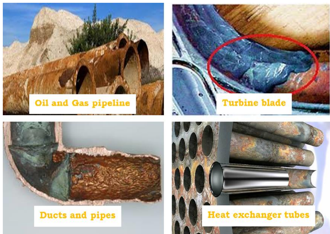
Fig. 1.1: Components suffering from material degradation due to erosion-corrosion.
