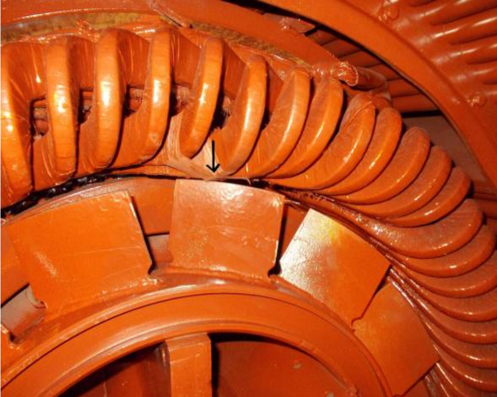
Figure 5.7: Pictorial view of rotor touching the stator winding
